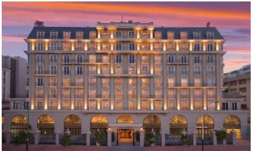
Window and Door Surrounds in Fibre Reinforced Concrete supplied and installed by Old World Concretes. Also precast concrete Balustrade supplied and installed.
